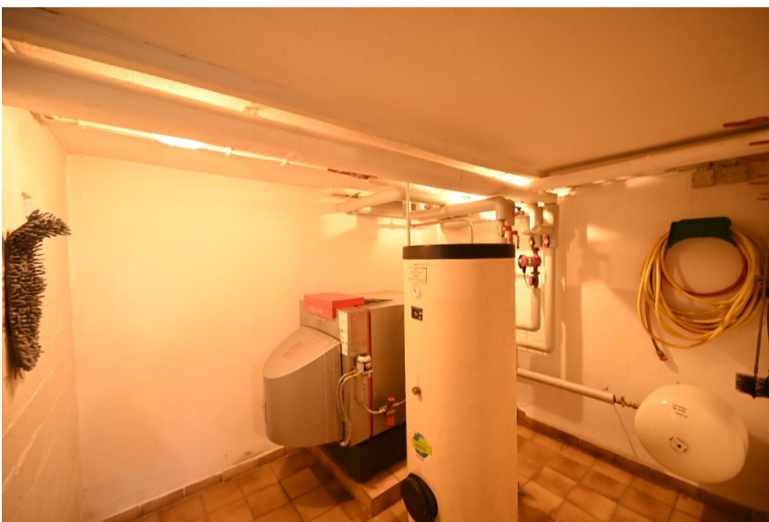
Heizung Fa. Viessmann
